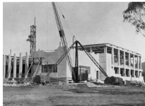
The construction of the Australian Institute of Anatomy. Courtesy of National Archives of Australia
